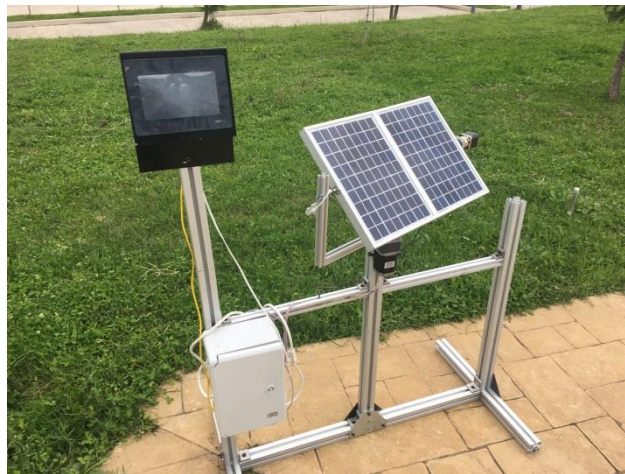
Figure 5. General view of the implemented solar tracking system.
